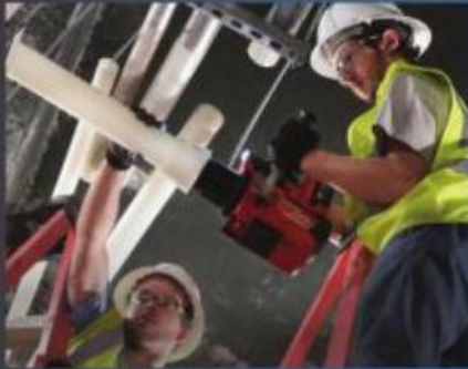
Commercial PEX plumbing
